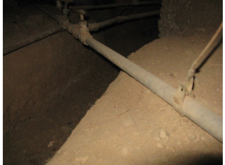
Unsupported supply line in crawlspace
