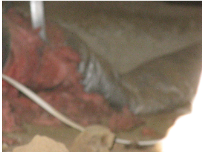
Crushed ducting in crawlspace
