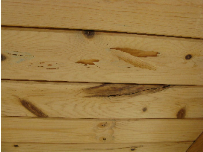
Pest damage at family room ceiling
